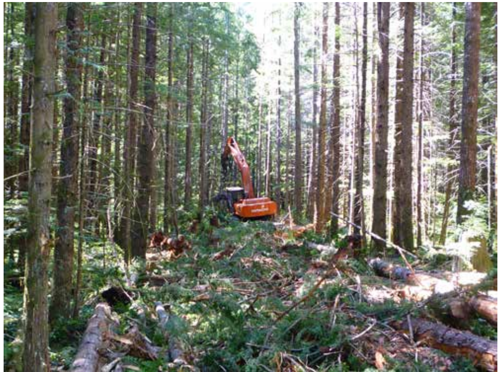
Excavator falling and processing wood in one of the thinning corridors to create a herringbone pattern to reduce wind throw
