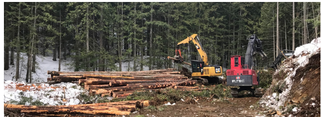
Winter logging on W1834 along Flowdown Trail, a part of Revelstoke Cycling Association’s Mount Macpherson trail network.
